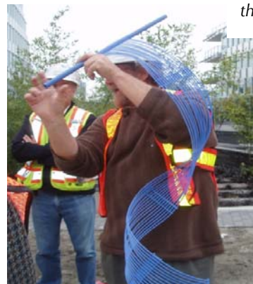
New hydronic radiant "capillary mat" system (pictured left) imported from Germany used on some of the buildings for radiant heating
